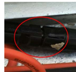
The cable is loose
